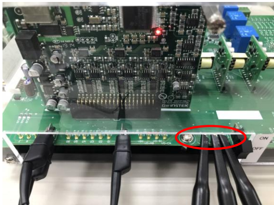
Figure 8.7 Oscilloscope test leads wiring
