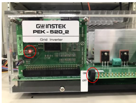
Figure 1.8 DSP normal status with light on
