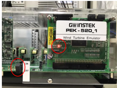
Figure 7.6 DSP normal status with light on
