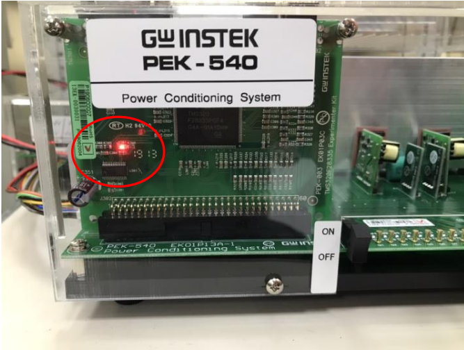
Figure 4.8 DSP normal status with light on
