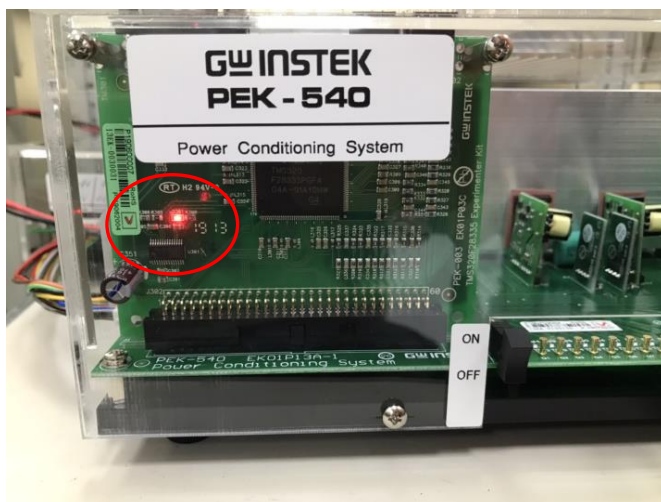
Figure 7.8 DSP normal status with light on
