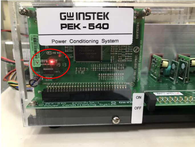
Figure 5.6 DSP normal status with light on
