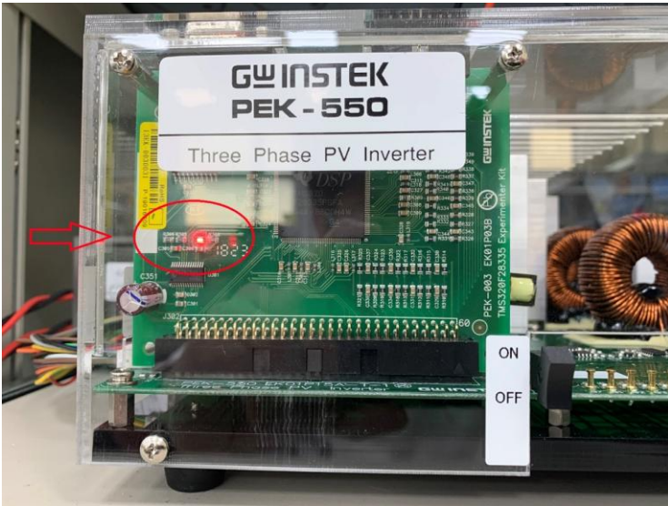
Figure 4.23 DSP normal status with light on
