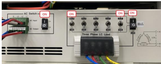
Figure 5.17 Fine tune load capacitor (in parallel 5uF)
